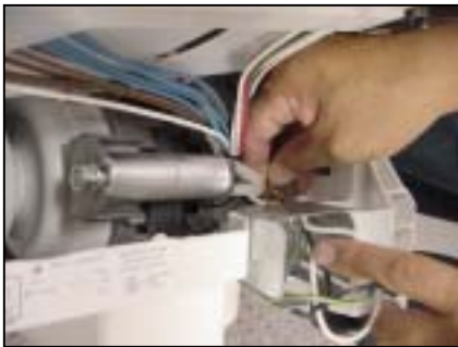
Pull wires from J-box
