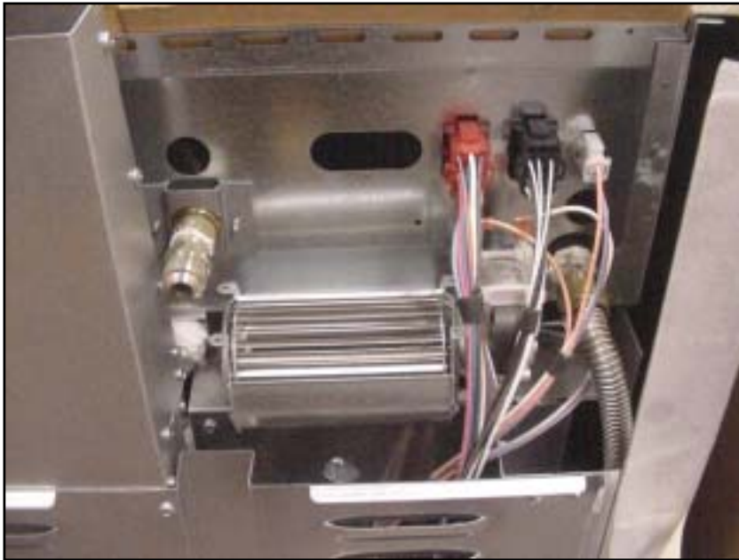
Rear of unit showing gas connection, cooling fan and moxex plugs
