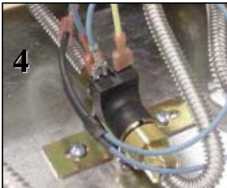
Solenoid gas valve receives 110 VDC from simmer controller through potentiometer contacts 1-5
