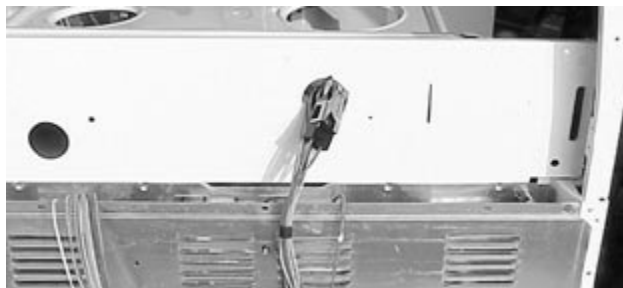
Hole in splash panel
