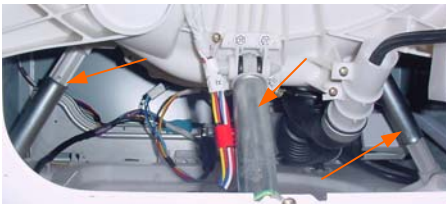
Dampers as seen from the back.
