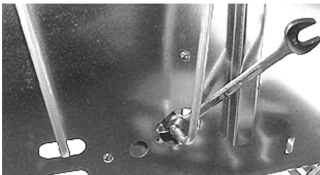
Disconnect tubing at back of safety valve
