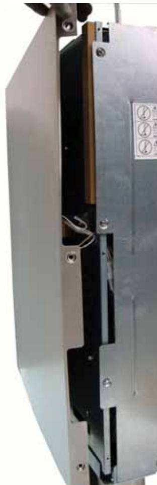
Panel Moved Out
